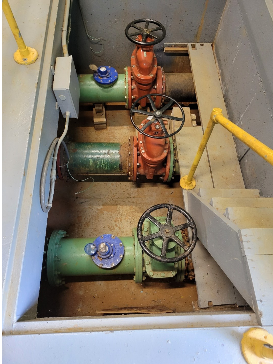
Two upper valves are new at the Ranney Well site.
