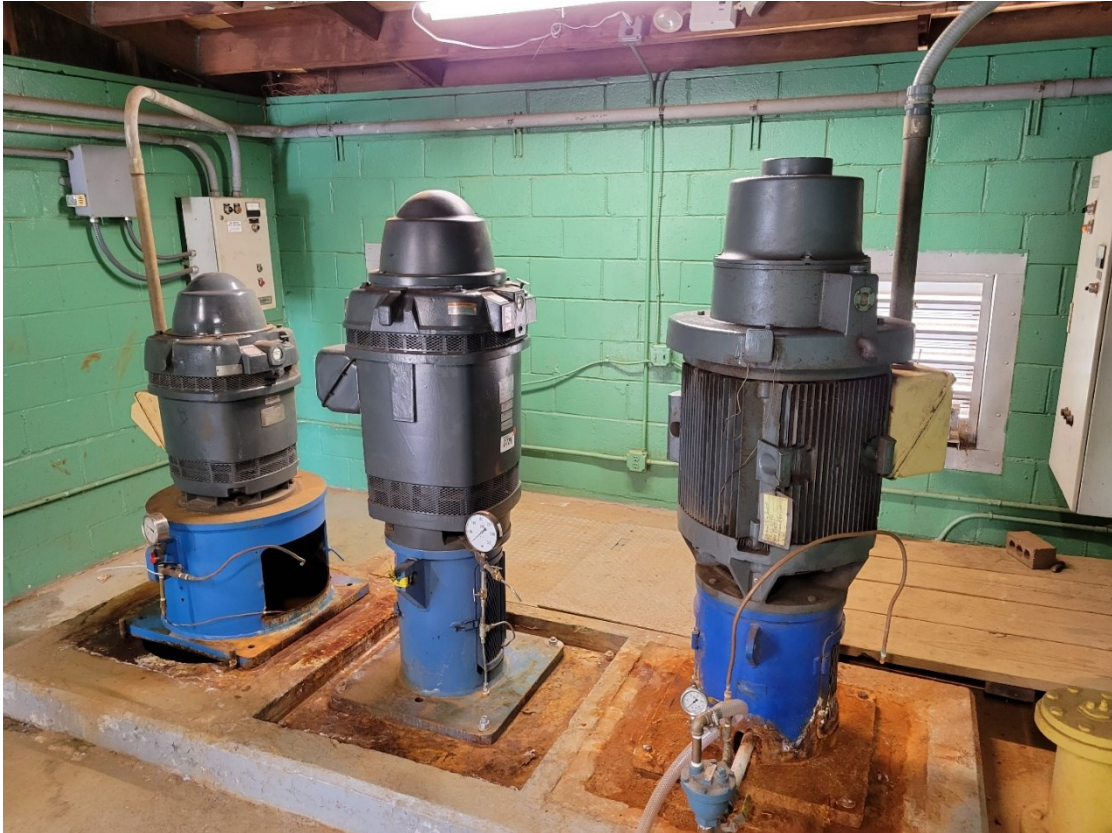
New motor at Ranney well being installed (middle pump). Pump capacities of the above pumps are Left to Right 2MGD, 4MGD, 4MGD.
