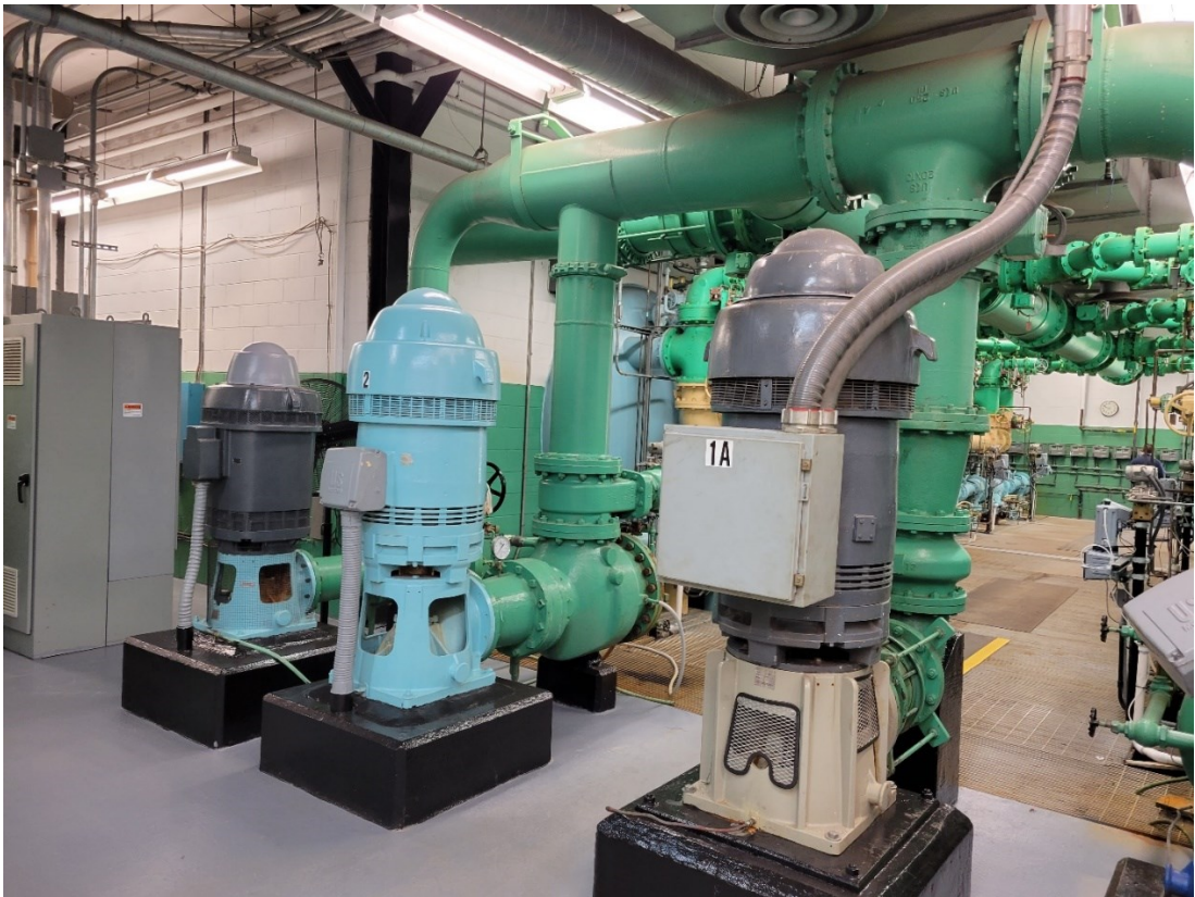
Treatment plant pumps, newest on the left.
