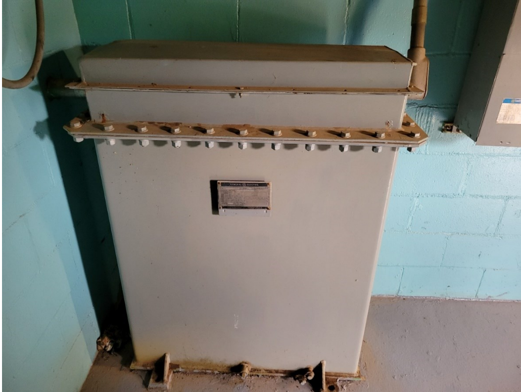
OLDER OIL FILLED TRANSFORMER (see plug on bottom for oil)
